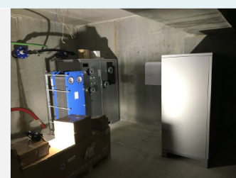
Figure 18: Heat pumps and heat exchanger Powerhouse before installation (October 2019).
