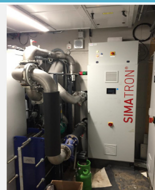
Figure 17: Heat pump and heat exchanger Sportscomplex (October 2018).
