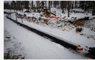
Figure 36: DH pipe, a "district level" size. Supply and return inside the same polyurethane insulation. Steel pipes.
